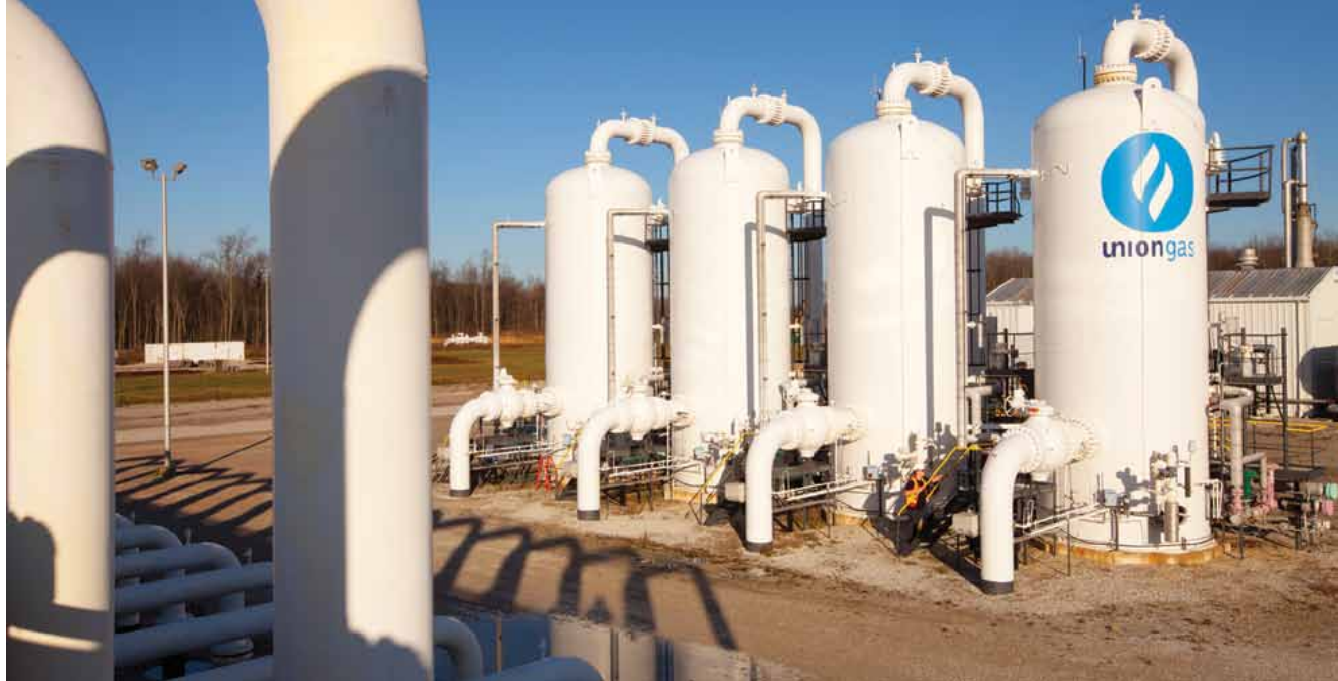
Natural gas storage facilities at Dawn, Ontario. Photo: Union Gas Limited
