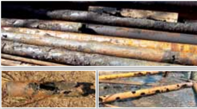
Steel casings recovered from orphan wells plugged by the Abandoned Works Program of the MNR, illustrating corrosion by exposure to sulphur water in subsurface aquifers.
