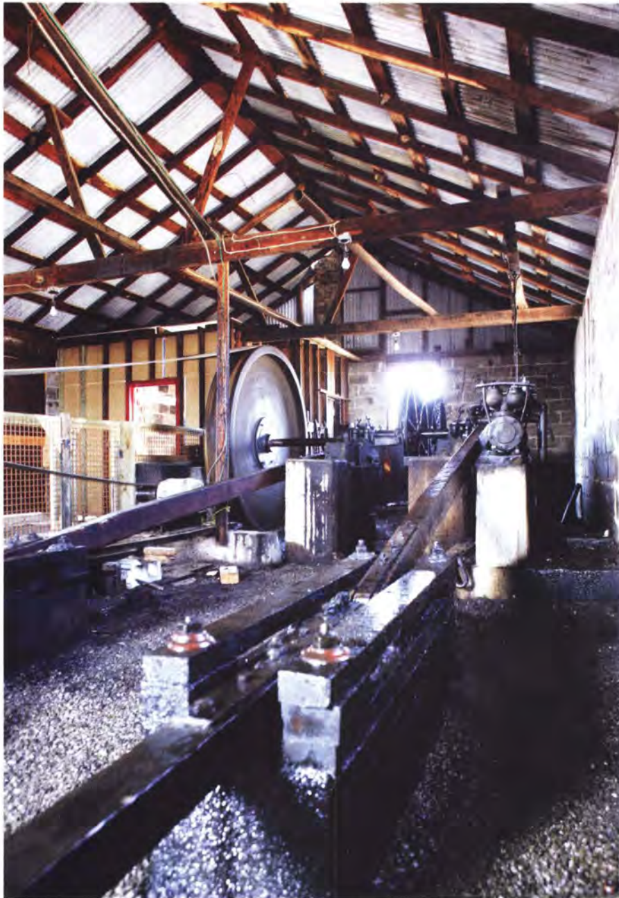
An electric motor powers Fairbank Oil's jerker-line system.
